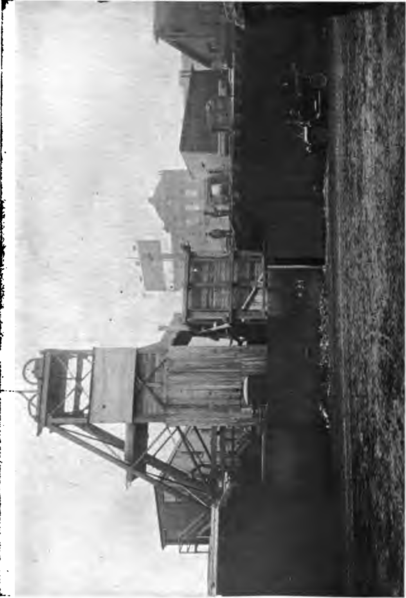
PLATE 226.—Contract 67. Shaft 19. Steel Headframe, Muck Bins, and Timber Deck at Shaft. Headframe boxed in for protection of men in shaft, and top protected by doors.
